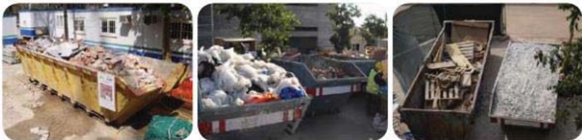
Figura 1.1. Separarea deșeurilor pe amplasament ( Sursă: Ilobe manual for drafting and implementing a construction and demolition waste management plan and good trade practices, Ilobe public company for environmental education, 2012)
